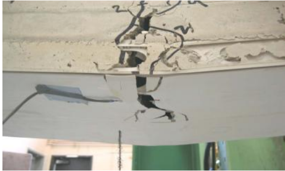
Typical Rupture of Octaform Panels
