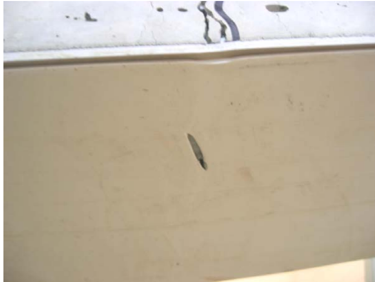
Figure 3.10 A crack in a tension panel in the Octaform-encased reinforced specimens
